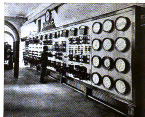
ELECTRIC SWITCH BOARD
