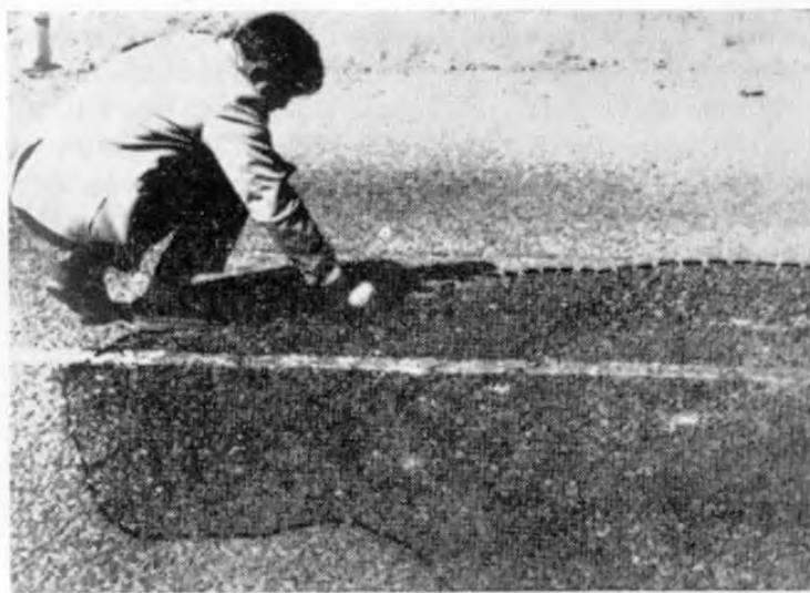
Photograph by courtesy of Die Vaderland, Johannesburg Outlined—the burnt tarmac patch
