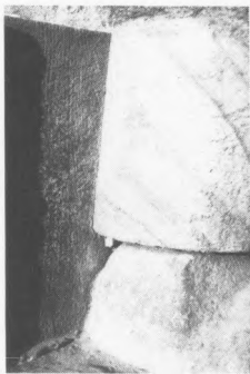
Fig. 10. Individual granite blocks of the skim have been carefully fitted to the limestone blocks of the core.
