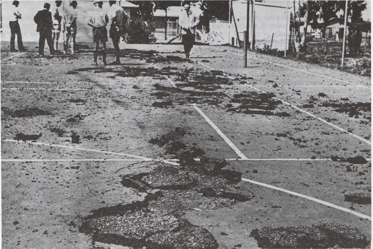
“Sucked Up” surface of tennis court showing extensive damage— at Rosemead, South Africa.
